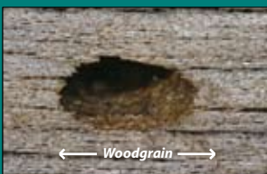
EHB exit holes always run with the grain
