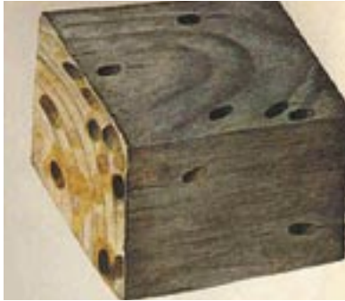
Off-cut of timber exhibiting oval-shaped exit holes caused by emerging adult beetles.
