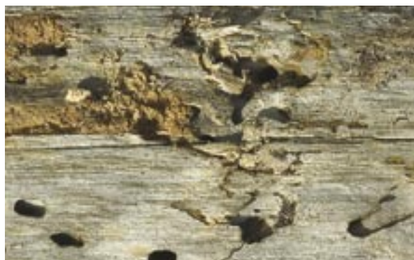
Damage to a log caused by the European House Borer.
