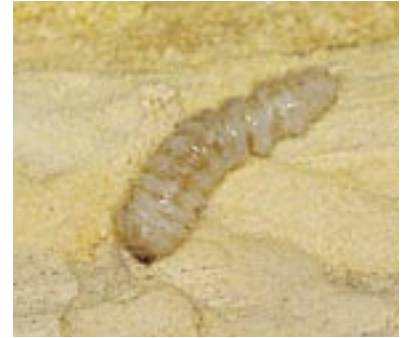
Exposed larvae boring through timber. – Picture not to scale (Clemson University USDA Cooperative Extension Slide Series)
