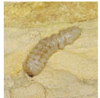
Exposed larvae boring through timber.
